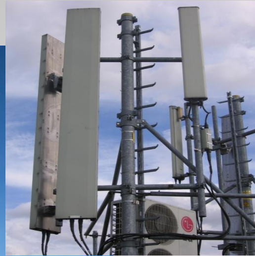
BTS antenna system
