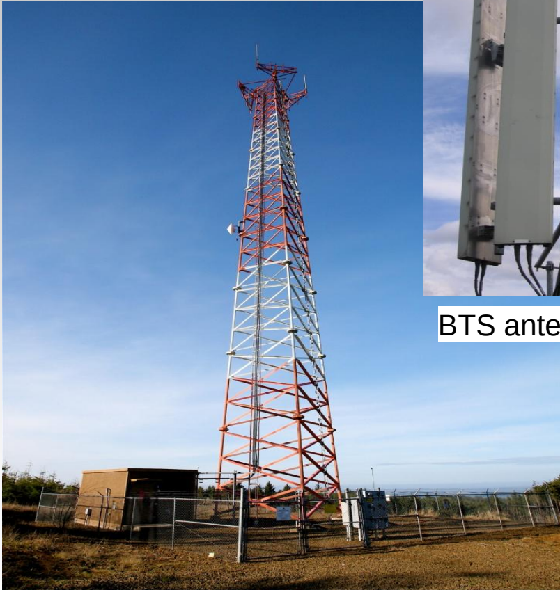
Typical BTS installation
