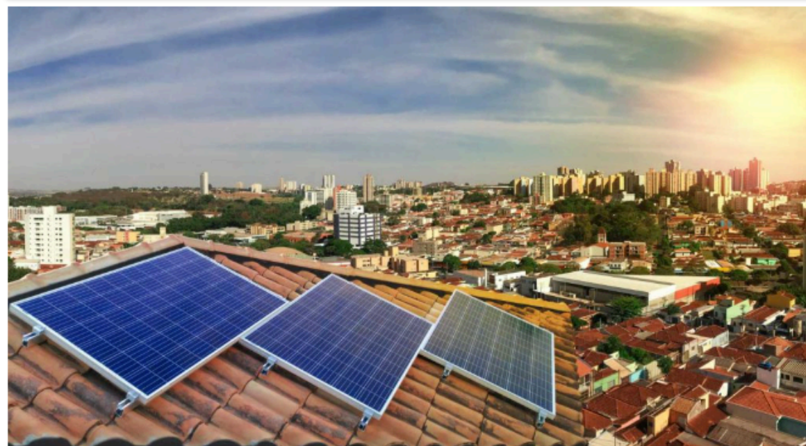
PV panels are installed on the rooftops of Santa Casa da Misericórdia buildings
