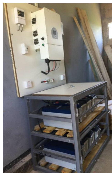
Figure 13: Inside the technical room. Note: Received from John, Personal communication, April 4, 2024.
